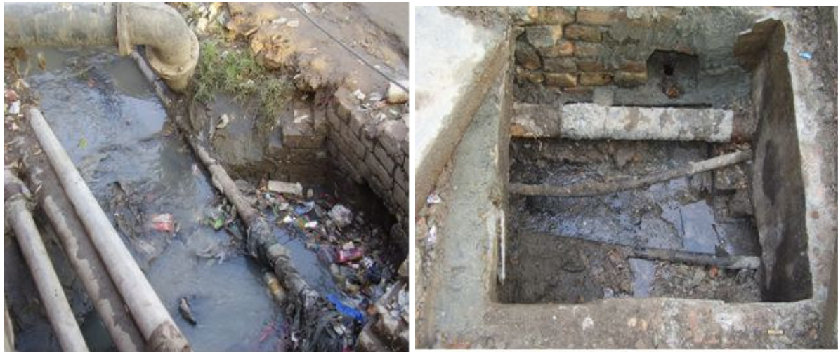
Fig. 8.1: Hand in gloves laying of drinking water distribution pipe lines with sewerage drains.
